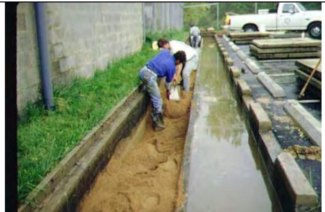
Routine cleaning of a perimeter or "Delaware" sand filter. This can be done from the surface, but deeper, vault-type filters will require confined-space entry procedures.
