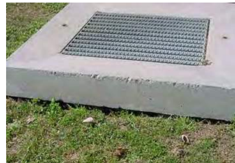
Water is “piping” down to the underdrain at the weak spot where the soil media meets the concrete overflow structure.
