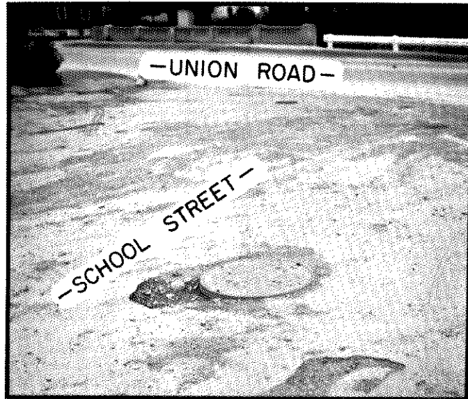
Photo No. 16. Manhole subject to surface flooding, about once in 5 years and causes basement flooding in the homes shown in photo no. 15. The homes would be subject to direct flooding about once in 20 years.
